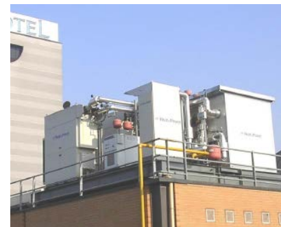
Hotel building with 130 kW e trigeneration plant, Milano, 2008
